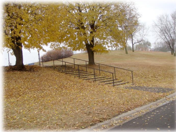
The staircase from the campus to Monroe Street NE is in poor condition
